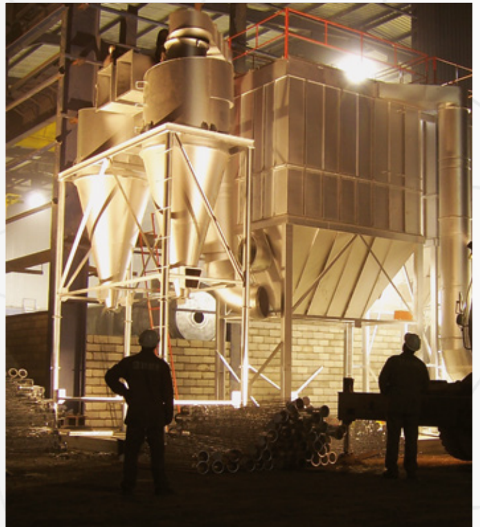
Capacity: 40.000 m 3 /h @ 450 mmWC • Motor Power: 75 kW Filtration Area: 432 m 2 • Project: Turkey • Sector: Steel Application: Dryer Filter
